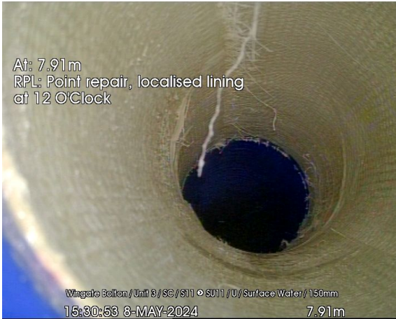
S11 - SU11_7-91m_153053.jpg, 00:00:38, 7.91 m Point repair, localised lining at 12 o'clock
