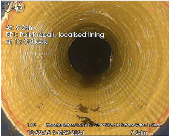
S7 - SU7a_9-24m_105235.jpg, 00:01:00, 9.24 m Point repair, localised lining at 12 o'clock
