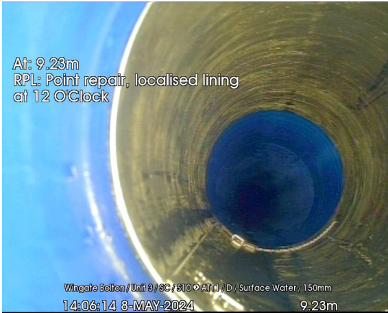
S10 - ATT1_9-23m_140614.jpg, 00:00:39, 9.23 m Point repair, localised lining at 12 o'clock
