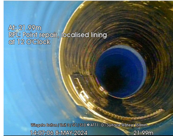
S10 - ATT1_21-99m_140706.jpg, 00:01:24, 21.99 m Point repair, localised lining at 12 o'clock
